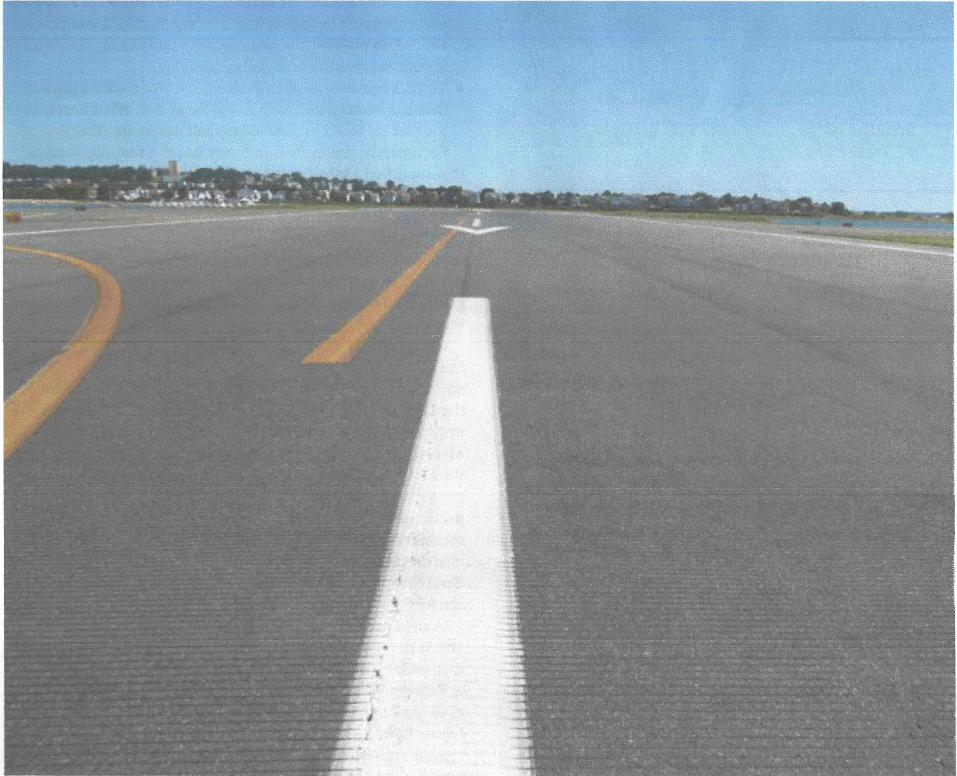
The Logan International Airport received its fuel-resistant asphalt pavement in 2004 and is still holding strong today. Photo courtesy of Axeon's Ron Corun.
